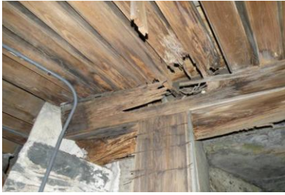
Fig. 19: Deteriorated girder and joists within a casemate.
