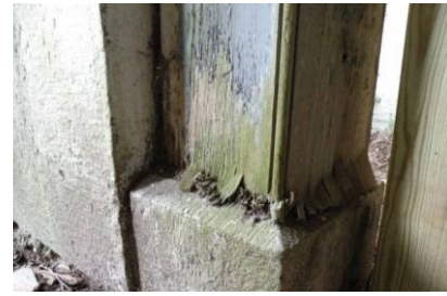
Figure 20: Brooming at the base of a column.
