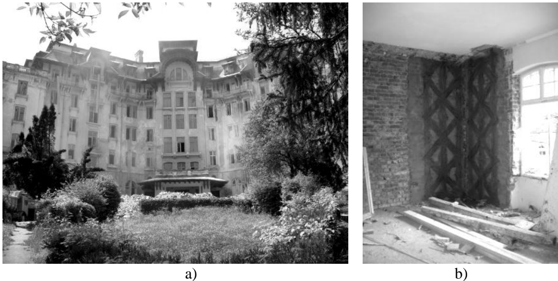
Fig. 5. Combined EBR and Central core strengthening techniques applied to: a) Palace Hotel, Govora; b) FRP EBR and central core reinforcements applied on an URM wall [20]
