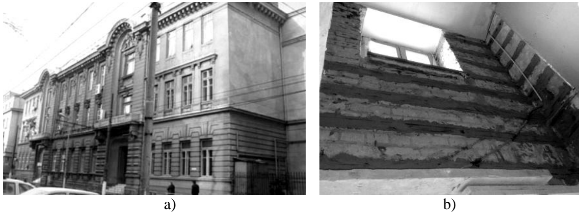
Fig. 2. FRP EBR strengthening technique applied to: a) Victor Slăvescu historical building; b) Laminates bonded on an URM wall [20]
